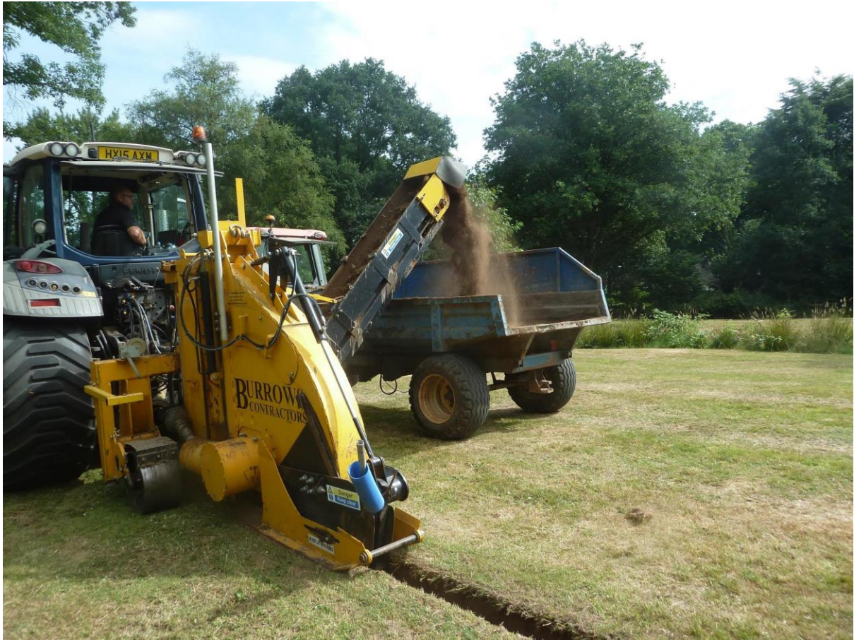
The trenching machine in operation – much quicker than digging them by hand!
